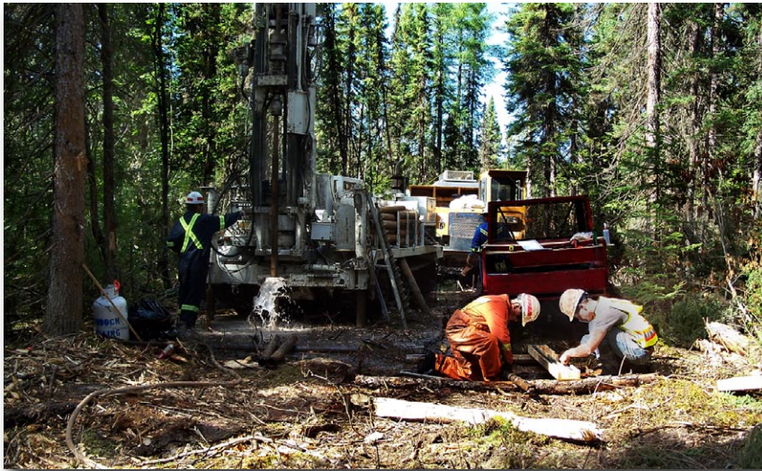
Preparing for borehole soil samples near the proposed project site for the geotechnical work.
