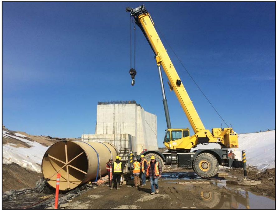
The first piece of the penstock for the project arrived on April 13, 2016.
